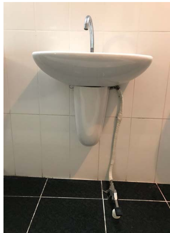
Figure 2. Pedal controlled lavatory faucets
