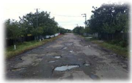
Figure 4. Lack of the water drainage from the road body
