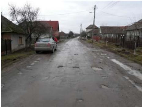
Figure 3. Lack of a rainwater collecting culvert
