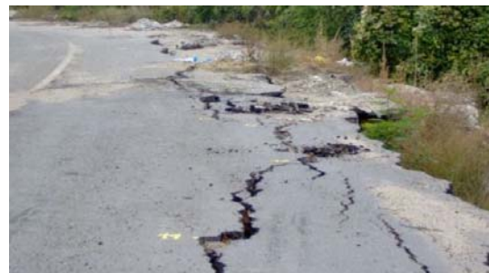
Figure 2. View of the crack length on the road
