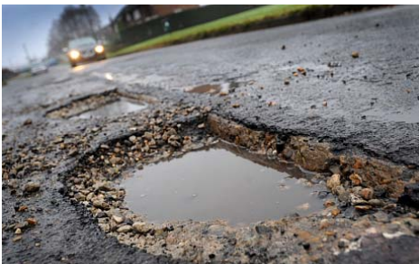
Figure 5. Lack of regular interventions to halt the progression of degradation
