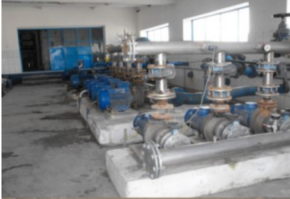
Figure 6. Vernesti pumping station
