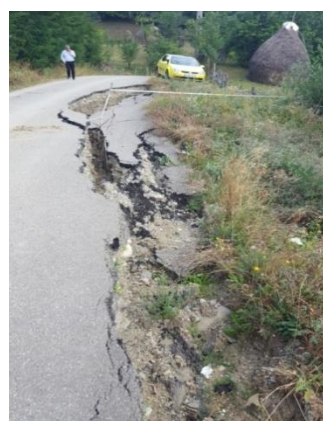
Figure 2. On site perspective after the landslide occurred
