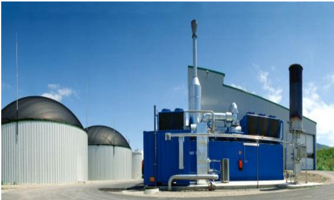
Figure 5. Heating system with biogas
